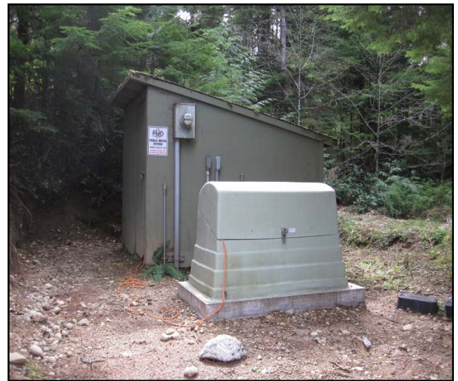
Vuecrest Well and Pump House
