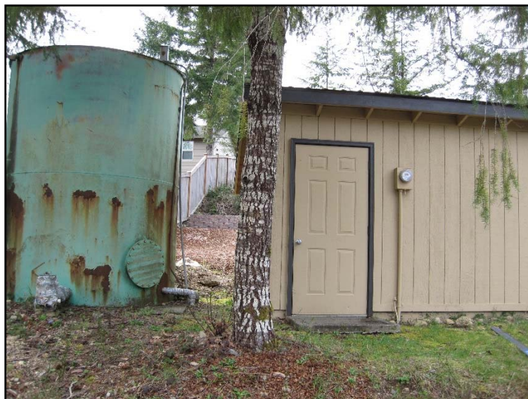
Reservoir and Booster Station
