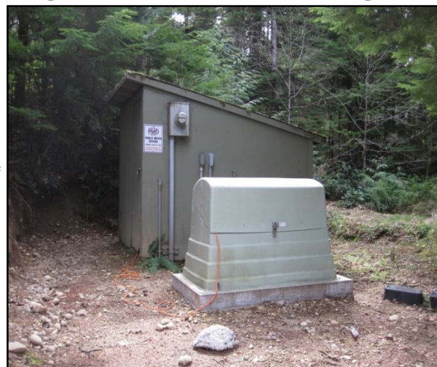
Well and Pump House
