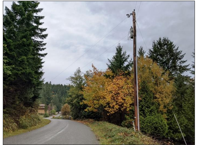
Figure A-11. View north to pole 3398 on Forest Drive in Triton.
