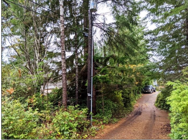
Figure A-24. View north to pole 3493 on unnamed road in Triton Head.
