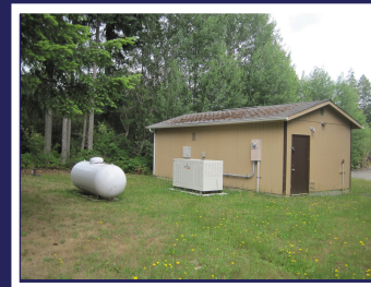
Back up generator
