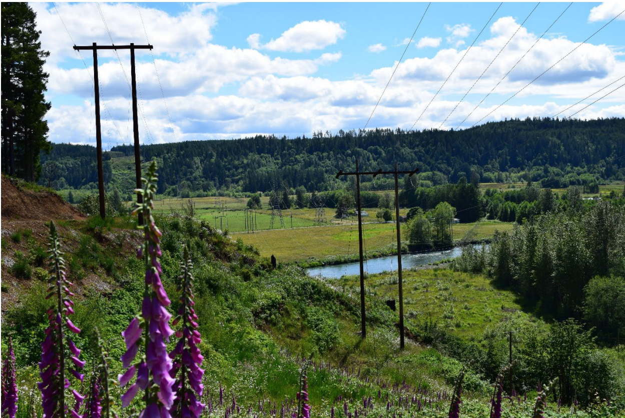
BPA AND MASON PUD 1 TRANSMISSION LINES, SKOKOMISH VALLEY, WA
