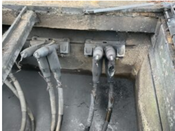
Underground power systems on the Tahuya Peninsula were damaged on Thanksgiving last year, leading to a power outage. (Photo courtesy of Mason County Public Utility District No. 3)
