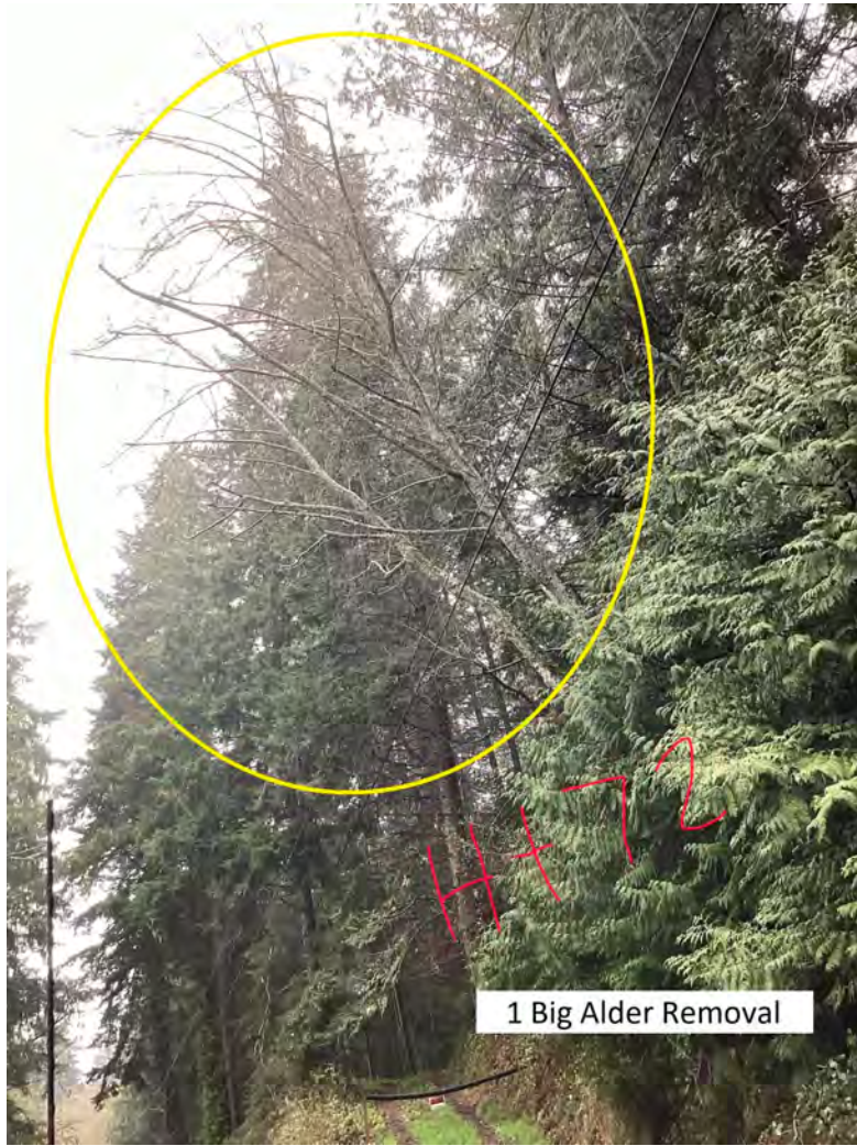
HT 72 Highway: SR101 Comments: 1 BIG ALDER REMOVAL Latitude: 47.551516 Longitude: -123.040049
