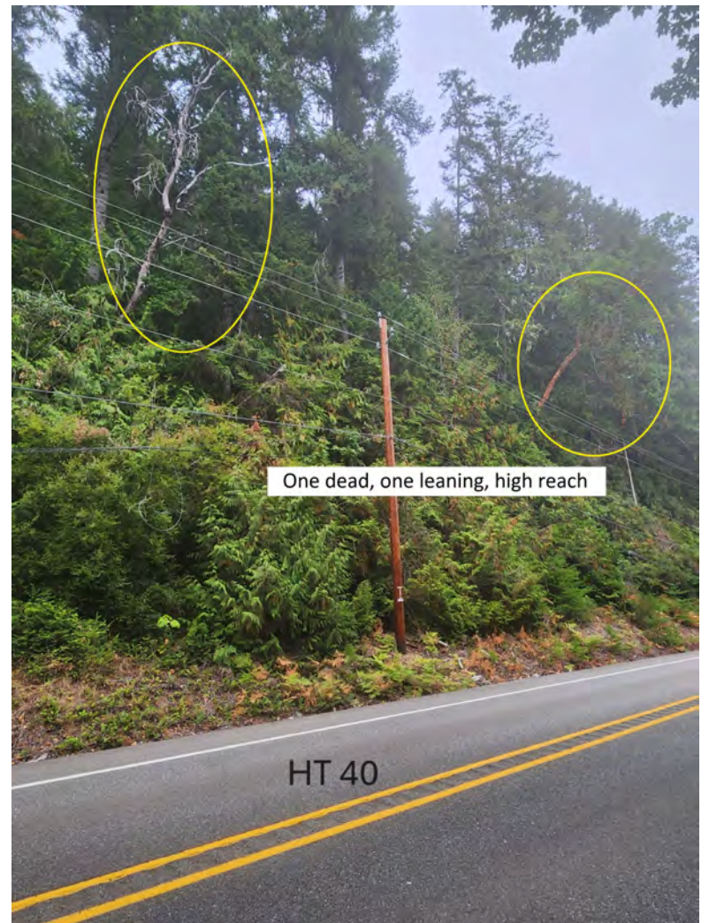
HT 40 Highway: SR101 Comments: ONE DEAD ONE LEANING, HIGH REACH Latitude: 47.60782917 Longitude: -122.9876964
