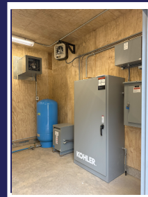
Electrical for Booster Station and Generator
