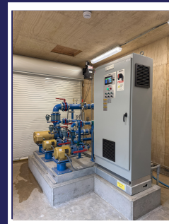
Booster Station and Control Panel
