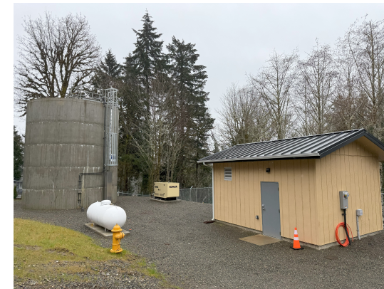
Agate Beach Reservoir, Booster Station Building, and Backup Generator
