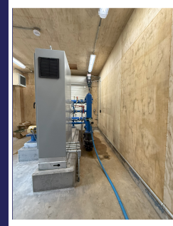
Back side of Booster Station
