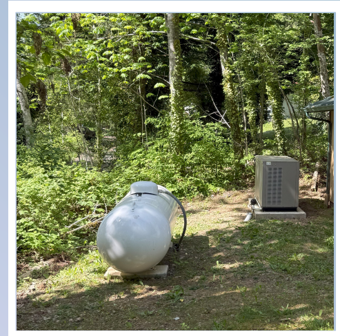
New Backup Generator and Propane Tank
