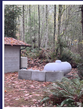
Propane tank and Generator
