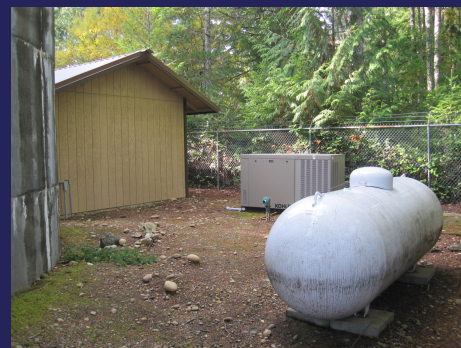
Backup Generator at the Booster Station
