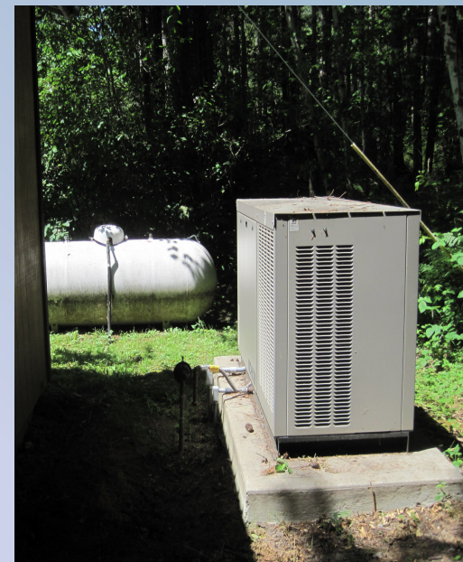
Generator and propane tank
